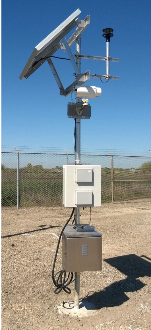
Laser detector, solar panel and circuit box
