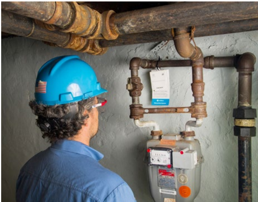
Residential methane detector installed in basement at gas meter location
